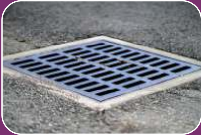
Storm Water Drainage Effective rainwater management
